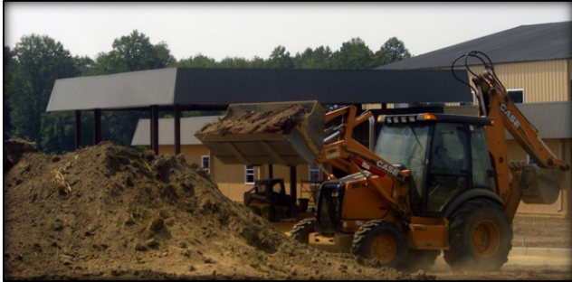
Upper: Stucco will be applied to the front soon. Lower: The mountain out front has become a mound!
